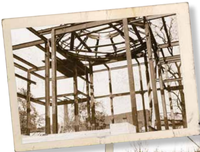
George A. Fuller & Company won the bid for construction of the American Institute of Pharmacy. Erection of the building took slightly more than one year with cost override because the government required APhA to use Danby Imperial Vermont Marble for the building facing.
